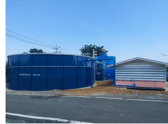
The Water Treatment and Water Supply System for Sawanpracharak Hospital (New Branch) Concession Period: 25 Years Capacity 2,400 m 3 /day
