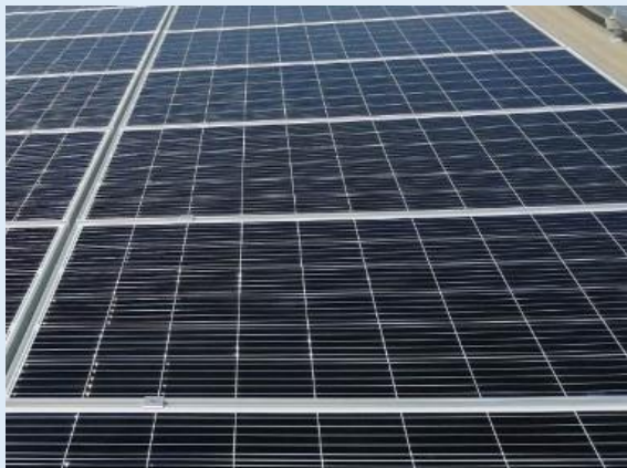
The Solar Power Purchase Agreement (Solar Rooftop) with Siam Quality Steel Co., Ltd. Contract Period: 10 Years Capacity: 0.6 MW
