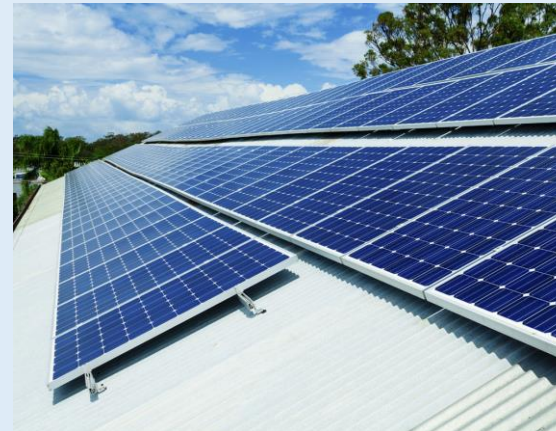
The Solar Power Purchase Agreement (Solar Rooftop) with Linh Gas Cylinder Co., Ltd. Contract Period: 10 Years Capacity: 1.0 MW
