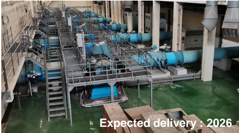
CSC of clear water tank at Bangplee water supply pump station and related works ; MWA
