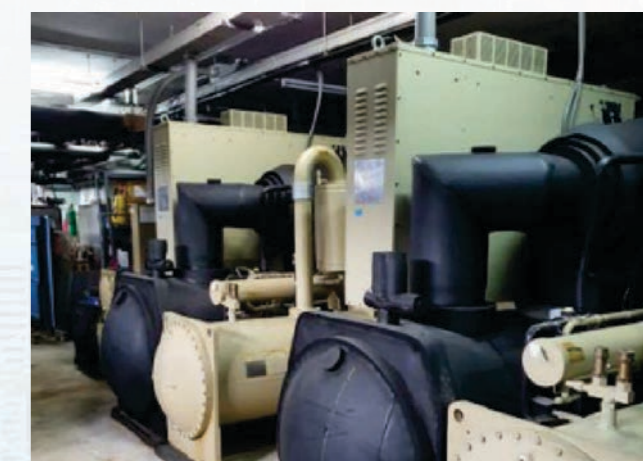
The smart chiller system installed at TEAM Building
