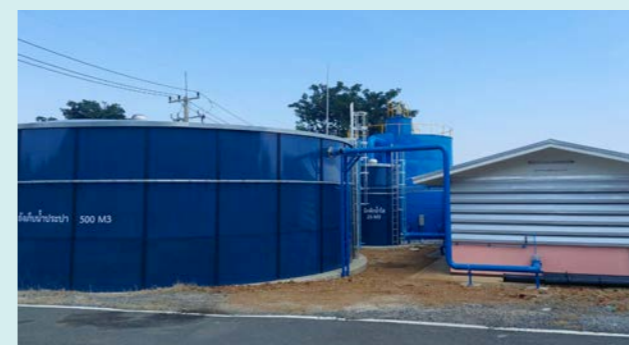
Water Treatment and Water Supply System for Sawanpracharak Hospital (New Branch)
