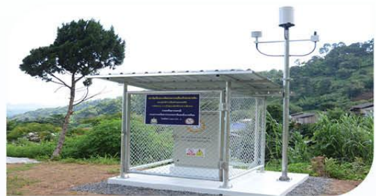
Procurement of a Landslide and Flash Flood Early Warning and Monitoring System (1 System) through Electronic Bidding (e-bidding): Department of Mineral Resources
