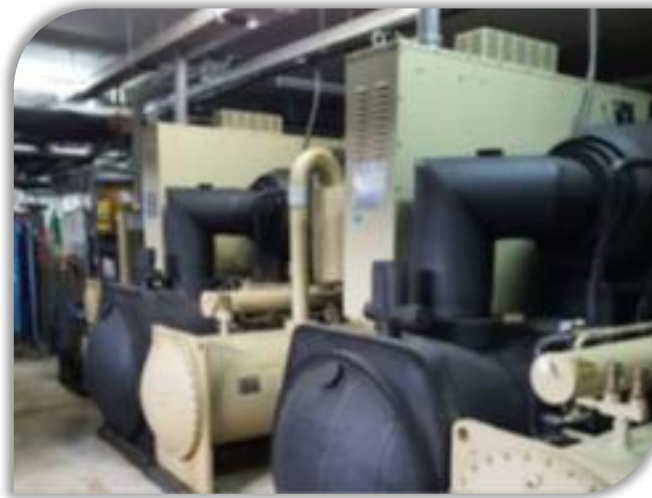
Image of the Smart Chiller system installed at the TEAM Building
